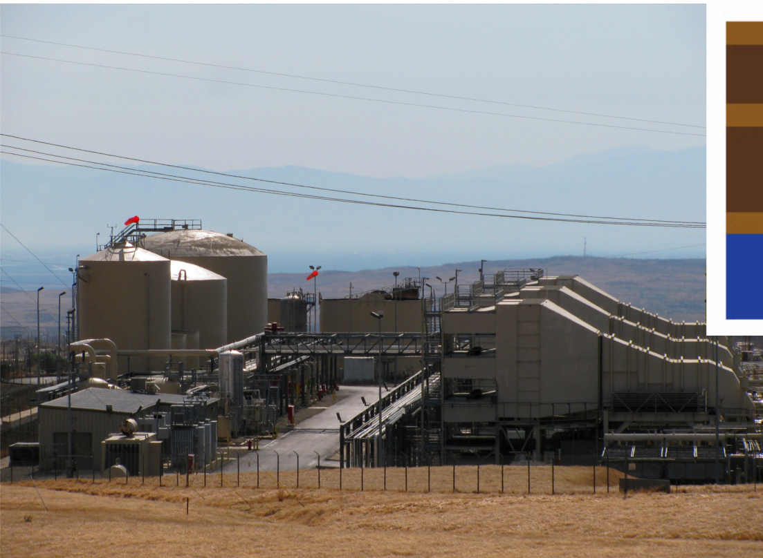
Steam Cogeneration Plant, Midway-Sunset Field
